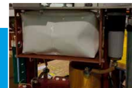
Protection of transformer oil - Electric -
